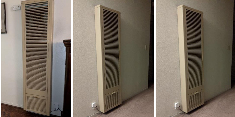
Figure 1: Existing Baseline Wall Furnaces in Hayward 3 (left), Hayward 4 (middle), and Oakland SFH (right)
