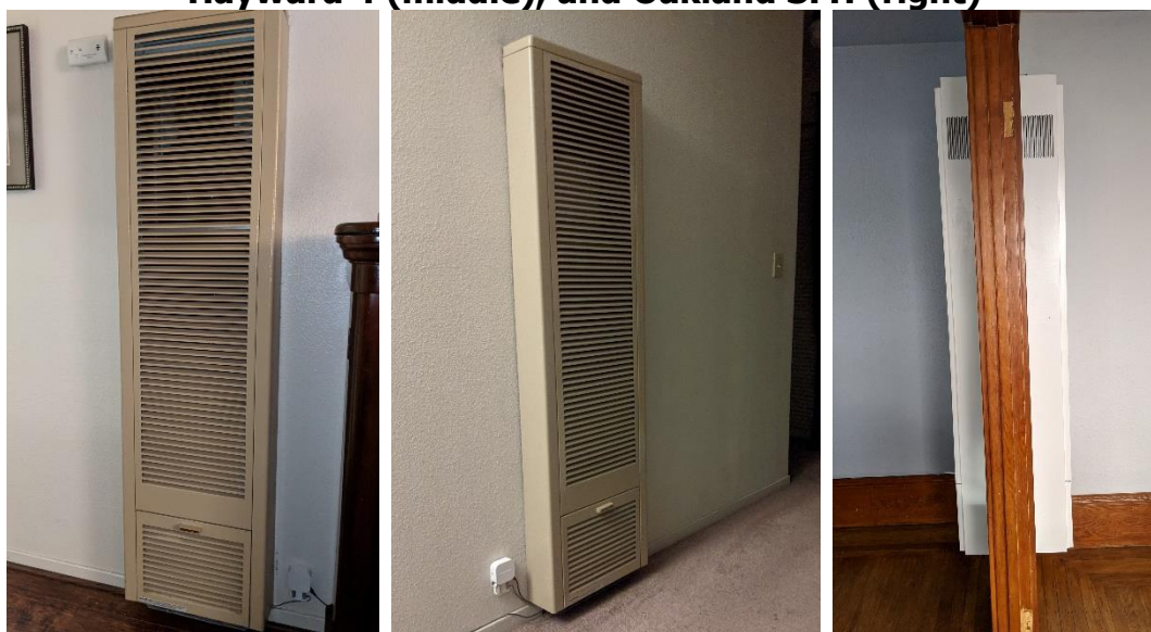
Figure 1: Existing Baseline Wall Furnaces in Hayward 3 (left), Hayward 4 (middle), and Oakland SFH (right)
