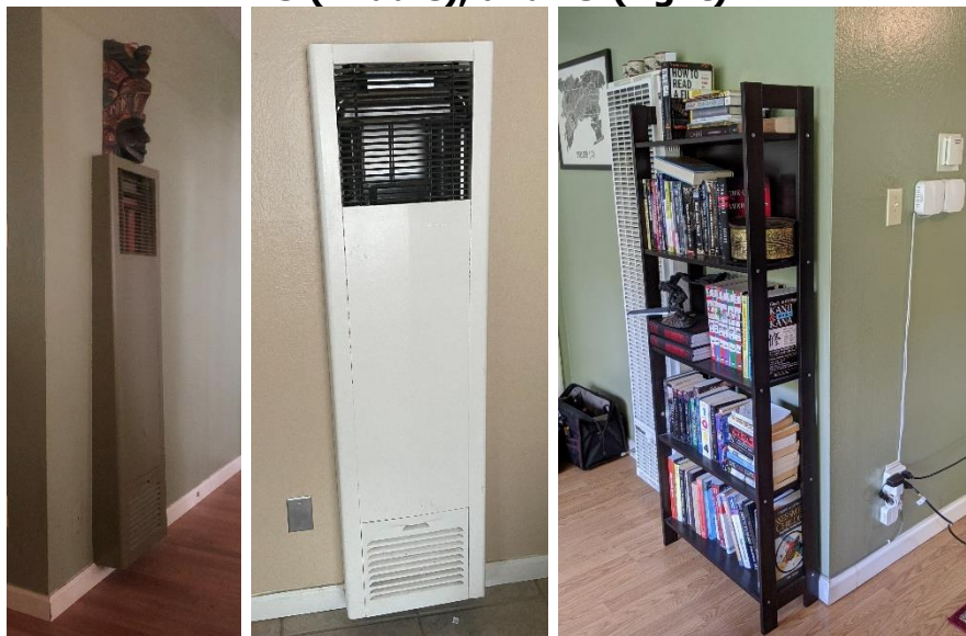
Figure 3: Existing Baseline Wall Furnaces in Sacramento Apartments 4 (left), 15 (middle), and 19 (right)
