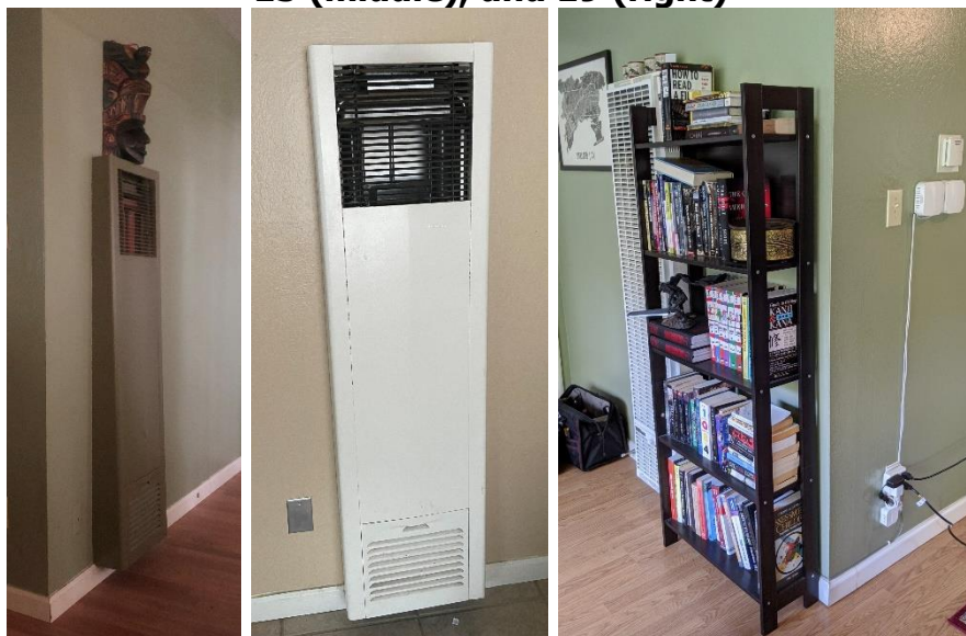
Figure 6: Existing Baseline Wall Furnaces in Sacramento Apartments 4 (left), 15 (middle), and 19 (right)
