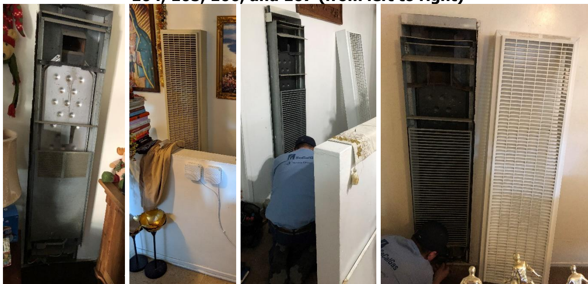
Figure 5: Existing Baseline Wall Furnaces in Los Angeles Apartments 104, 105, 106, and 107 (from left to right)
