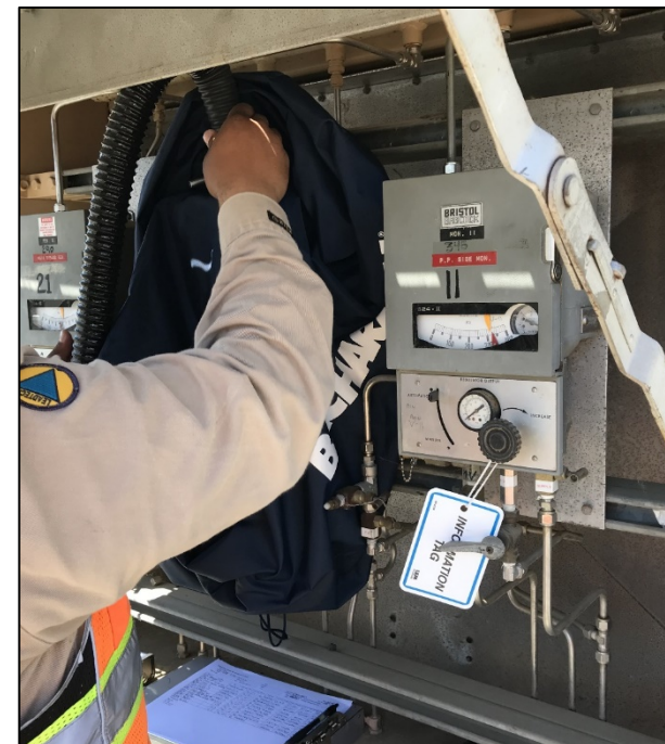
Continuous bleed controller at SP3 L-191 X-tie.
