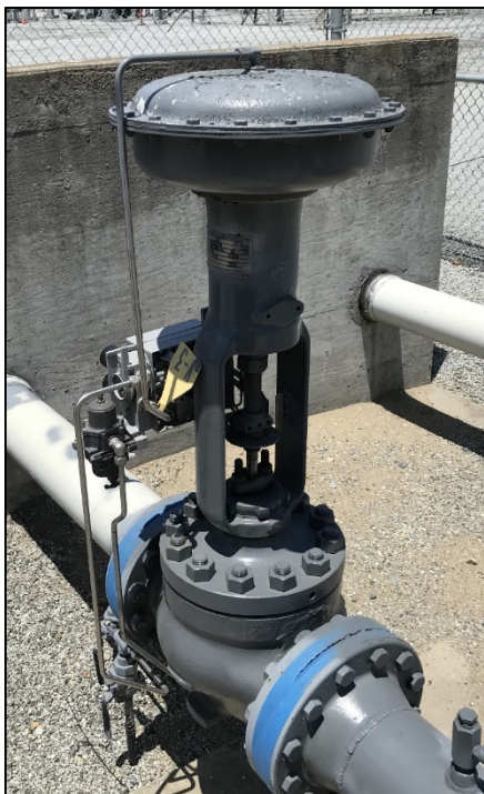
Continuous bleed regulating valve at California St.
