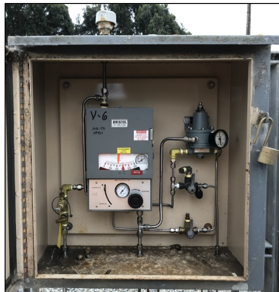
Continuous bleed controller at Harkins Rd.
