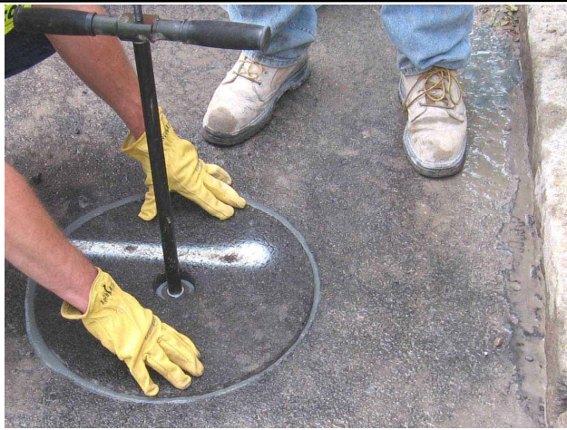
After the bonding material has been poured into the hole, the core is reinstated and carefully adjusted to be level with the rest of the pavement.
