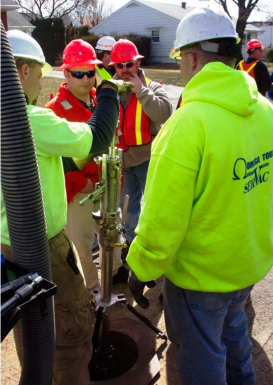
Above: Omega Tools (OTI) elevated pressure service abandonment equipment in the field at UGI.
