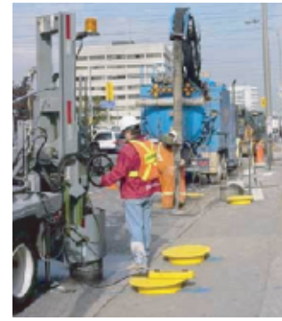
In May 2004, Robert B. Somerville undertook a large gas rehabilitation job on a busy, mixed residential and commercial arterial roadway in Toronto. Road coring and permanent pavement restoration was used.
