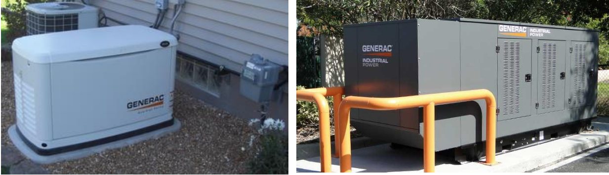
Figure 16: Example Residential and Commercial/Industrial Natural Gas Generator Sets
