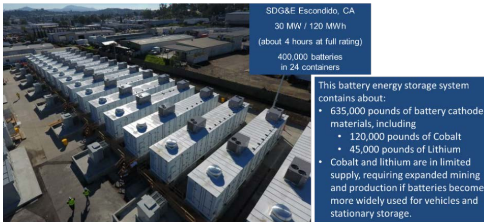
Figure 12: Example Large-Scale Battery Energy Storage System
