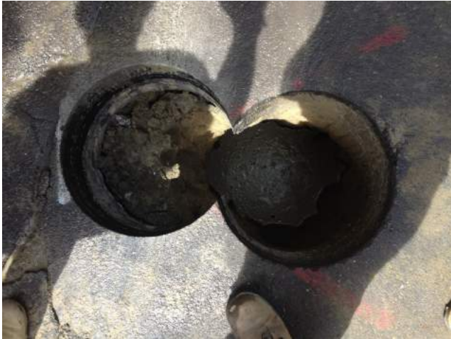
Two 18" diameter cores are cut to allow for greater access to buried facility
