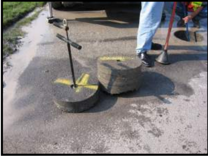
The Core shown above has been removed from the roadway. The layers of the core have separated. This is a delaminated core.
