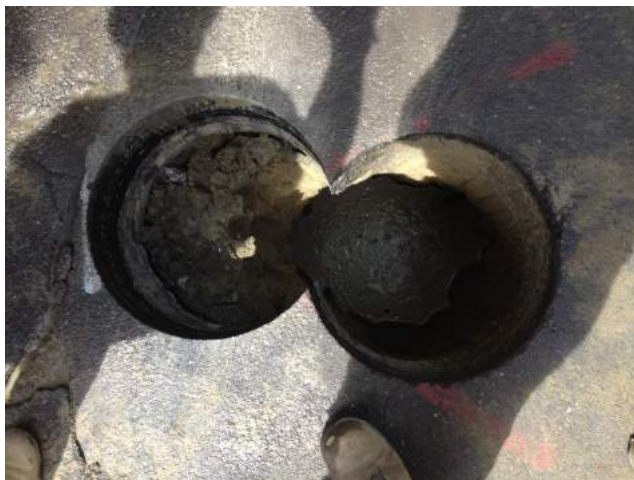
Two 18" diameter cores are cut to allow for greater access to buried facility
